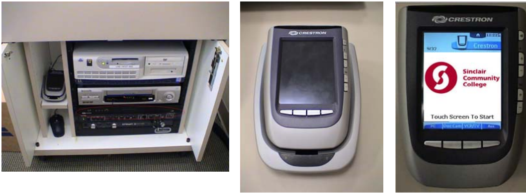
Figure 4-24. Podium equipment (left), Crestron control unit (center), and sample touch panel screen (right).
